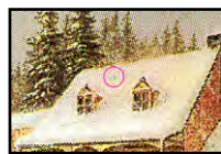
Pos. 45 Blue hole in roof
